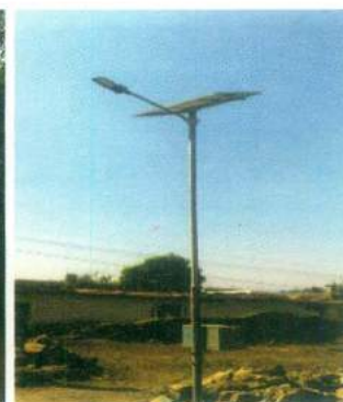
Solar Street Light
